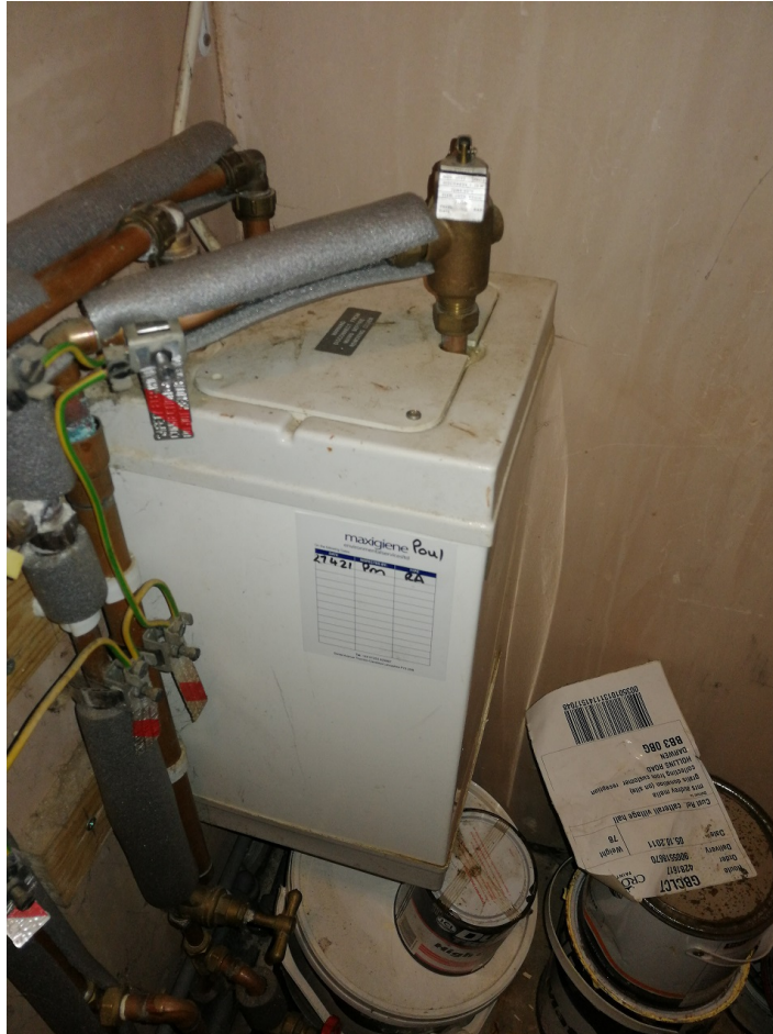
POU Water Heater 01
